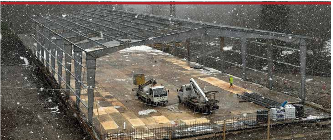
Warehouse - Central Asia
