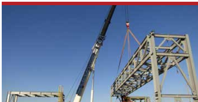
Pipe Racks - Saudi Arabia
